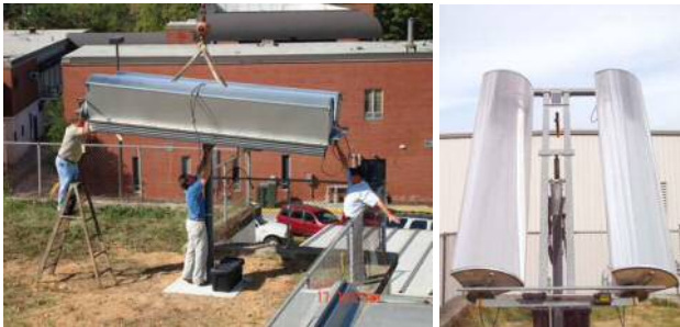
Fig. 5. Entech Solar SunLine installed at Auburn Univ.
